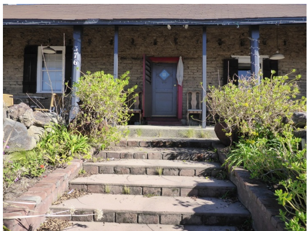
Cayetano Juarez Adobe, Napa, Napa County Avenue and Silverado Trail in the city of Napa, surrounded by commercial properties.
